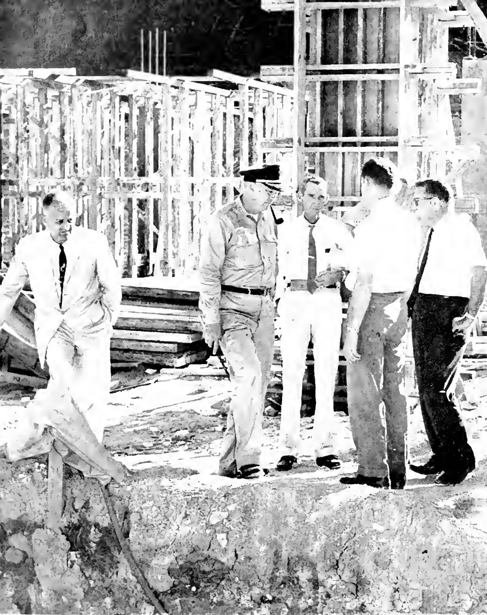
General Wilson at Gorgas Hospital project with Engineering and Construction Bureau Director Matthew C. Harrison, far left, Canal engineers, and others in tour party.
